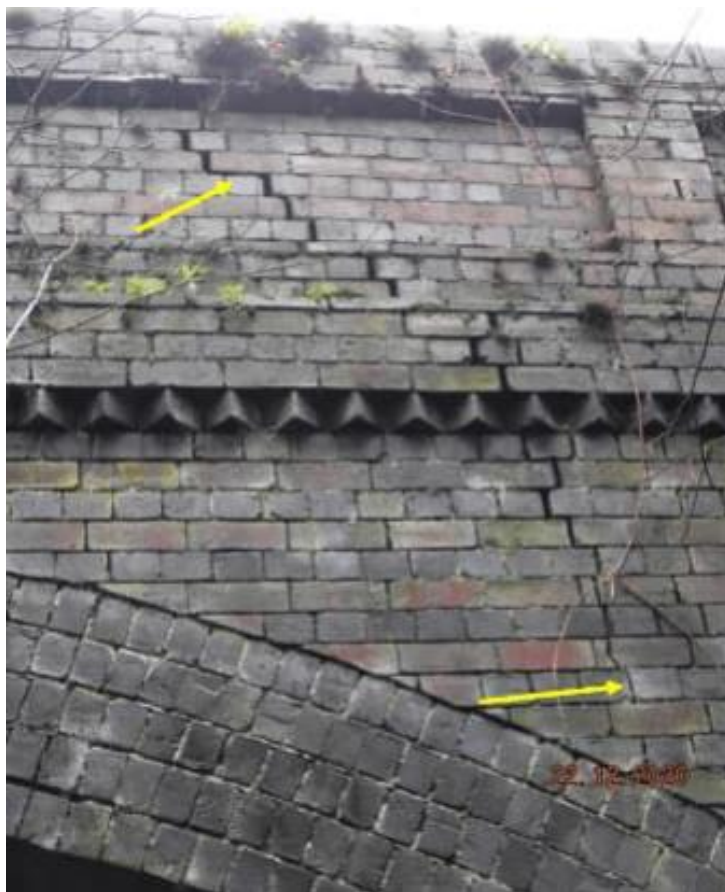
Plate A-6. Detail of vertical fracture in the north eastern elevation spandrel and parapet
