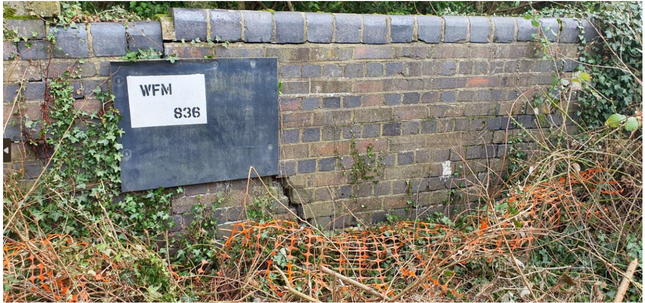
Plate A-5. View of the crack in the parapet wall of the bridge
